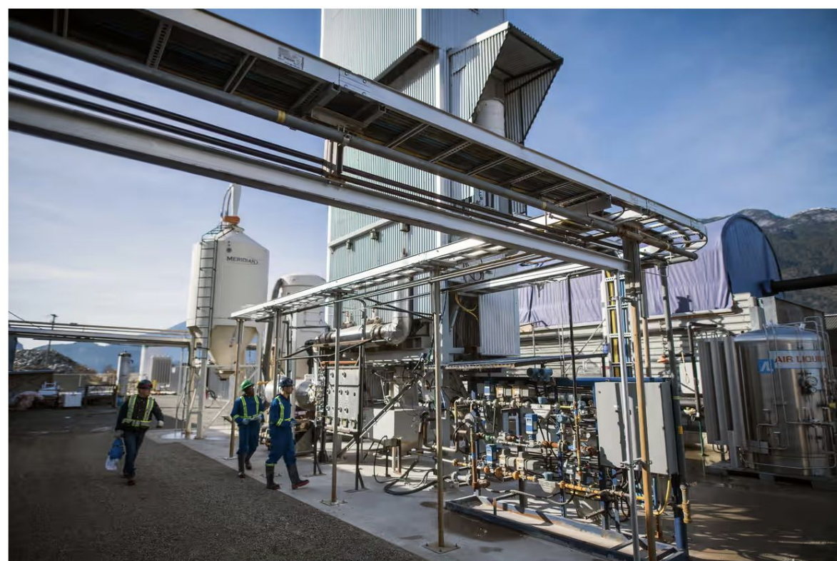
A direct air capture system at the Carbon Engineering pilot facility in Squamish, British Columbia, Canada. Photograph: Bloomberg/Getty Images
