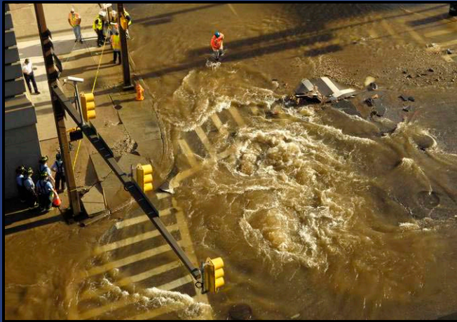
Water main break
